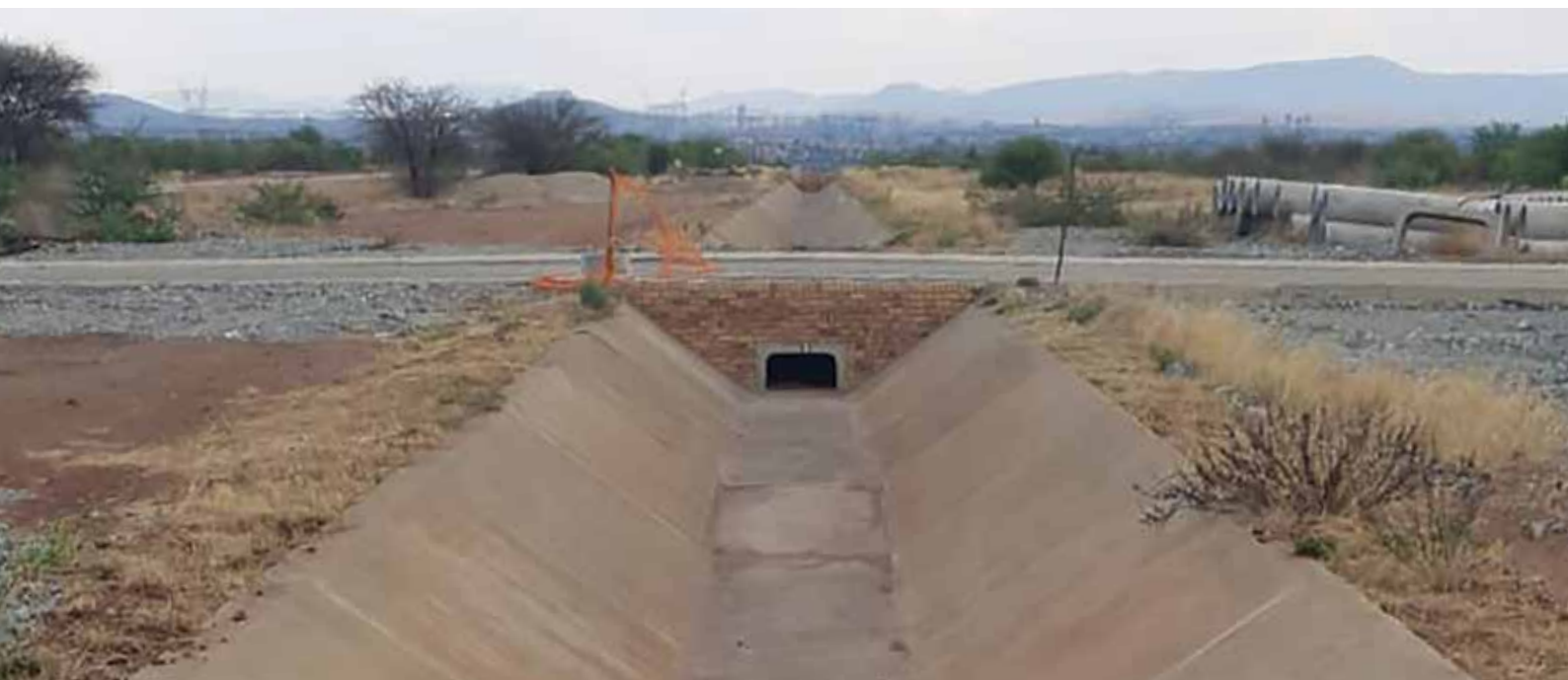
Storm water channel at BPM
