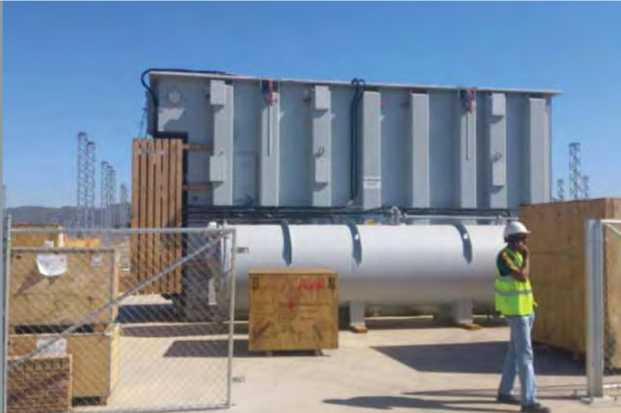
Figure 7: 500MVA Transformer at the Ngwedi substation (Courtesy of Eskom)
