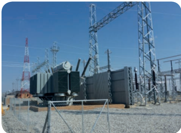
500 MVA transformer at the Ngwedi Substation
